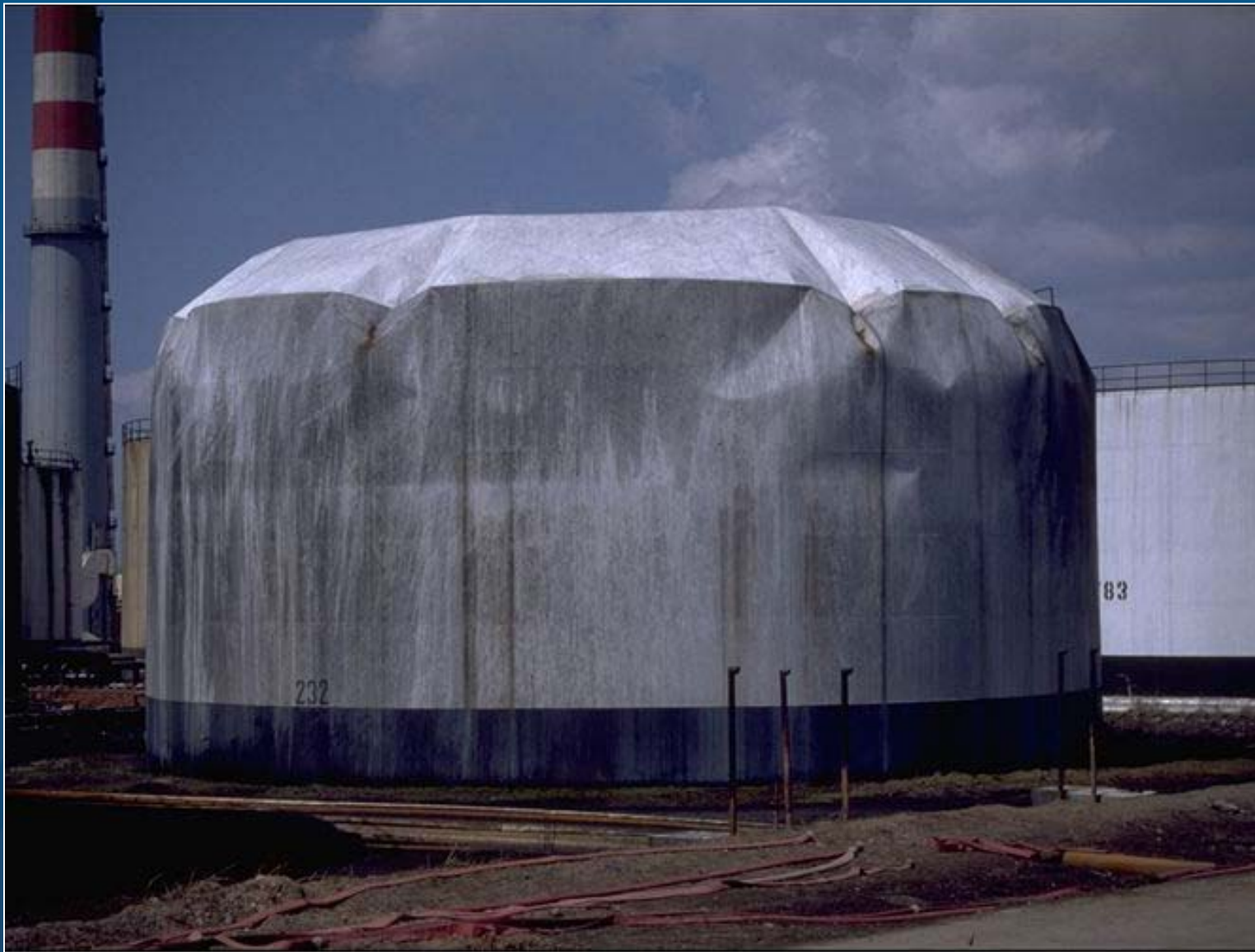
Roof damage in tanks due to liquid slashing
